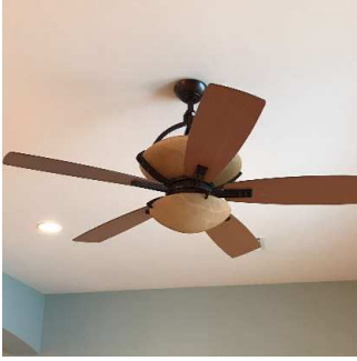
Ceiling Fan 09/14/2018 4:36 PM
