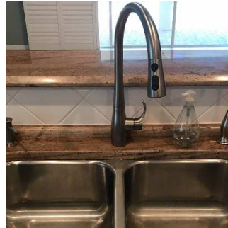
Sink / Faucet (1/3) 09/14/2018 4:40 PM
