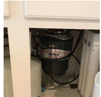
Sink / Faucet (2/3) 09/14/2018 4:40 PM
