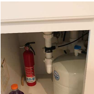
Sink / Faucet (3/3) 09/14/2018 4:41 PM
